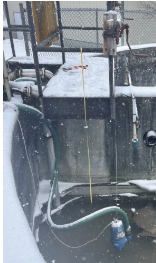
Decant pump (blue, bottom right) attached to a winch (top right).
