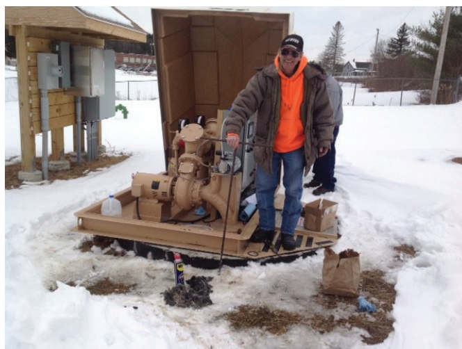
Buddy Ball uses a curb stop screw auger tool to remove a blockage.
