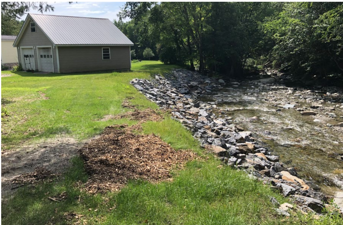
After EWP repairs, the streambank has been stabilized to prevent further bank erosion and danger to the buildings.
