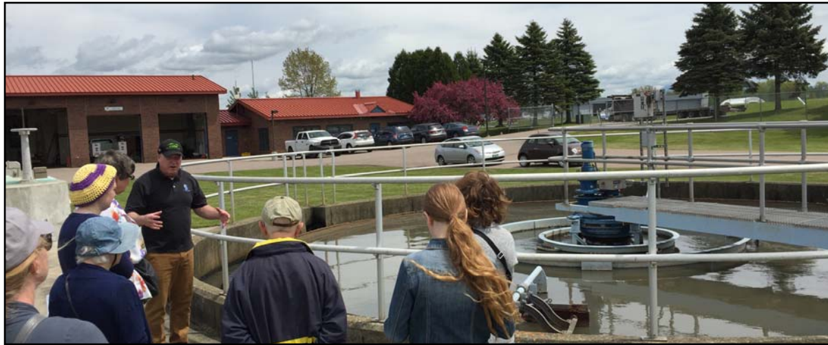
Bob Fischer, Water Quality Superintendent, conducts a tour of the South Burlington wastewater treatment facility on Water Quality Day, Thursday, May 30th, 2019
