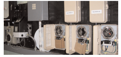
This bank of timers controls the aerators.
