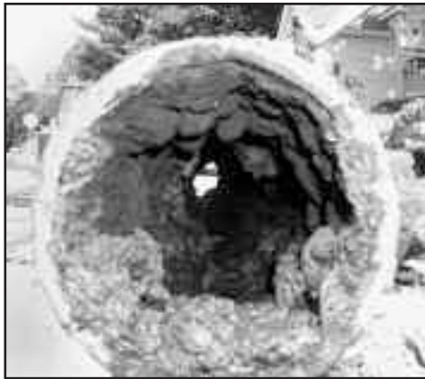
Do your water mains look like this after 112 years of service? (Photo courtesy of Dick Kilhart.)
