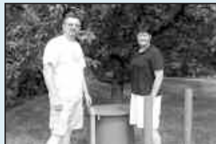
Kevin Colby stands with Paula Jackson outside of the water storage tank inspection hatch at the Waterford School in Waterford, Vermont. (Photo by Elizabeth Walker.)
