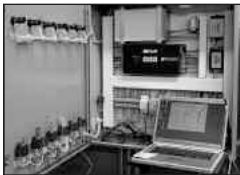
This SCADA system controls and monitors two well fields (total of 5 wells), two elevated storage reservoirs, a booster pump station, and incorporates some radio communication as well. Although this panel is up on a mountainside, the staff can remotely control and monitor the entire system from their office or home. (Photo courtesy of Ron Gehl, P.E., EOS Research)
