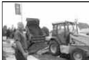
"That'll stop that leak!" Circuit Rider Jay Matuszewski is on the scene after a hydrant in Lancaster, New Hampshire was struck by a truck in the wee hours of the morning.
